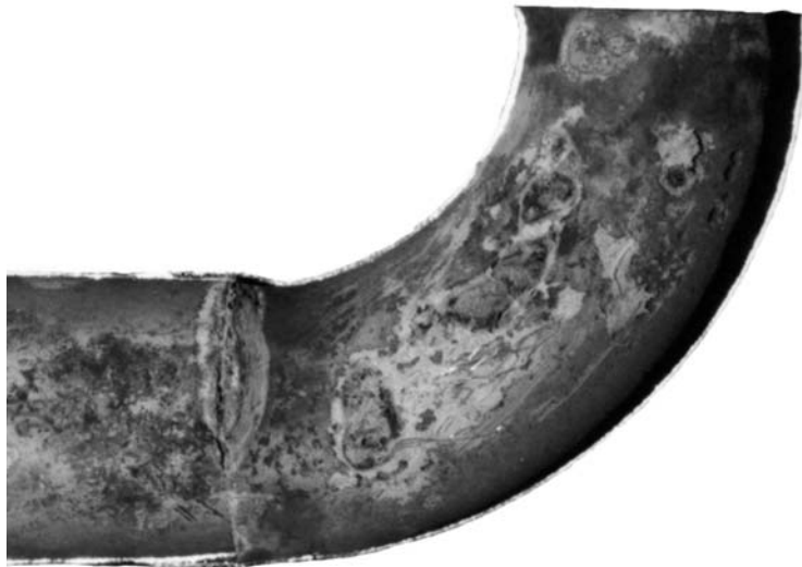
Figure 2. Copper pipe showing erosion-corrosion at start of bend
