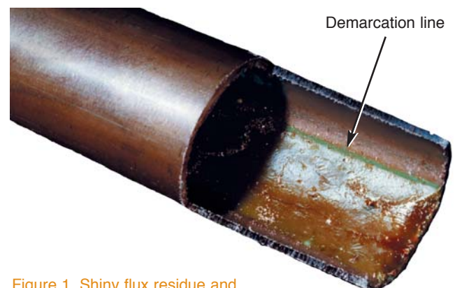
Figure 1. Shiny flux residue and demarcation line showing that the pipe was half filled
