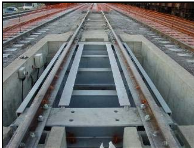
Figure 5.2.2.3 Typical conventional weighbridge 80 t capacity, 4 m long
