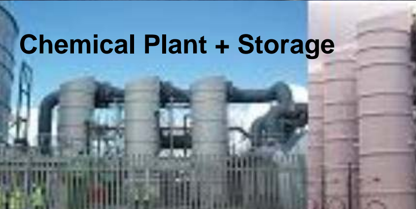
Chemical + Water Treatment Over 30 year service
